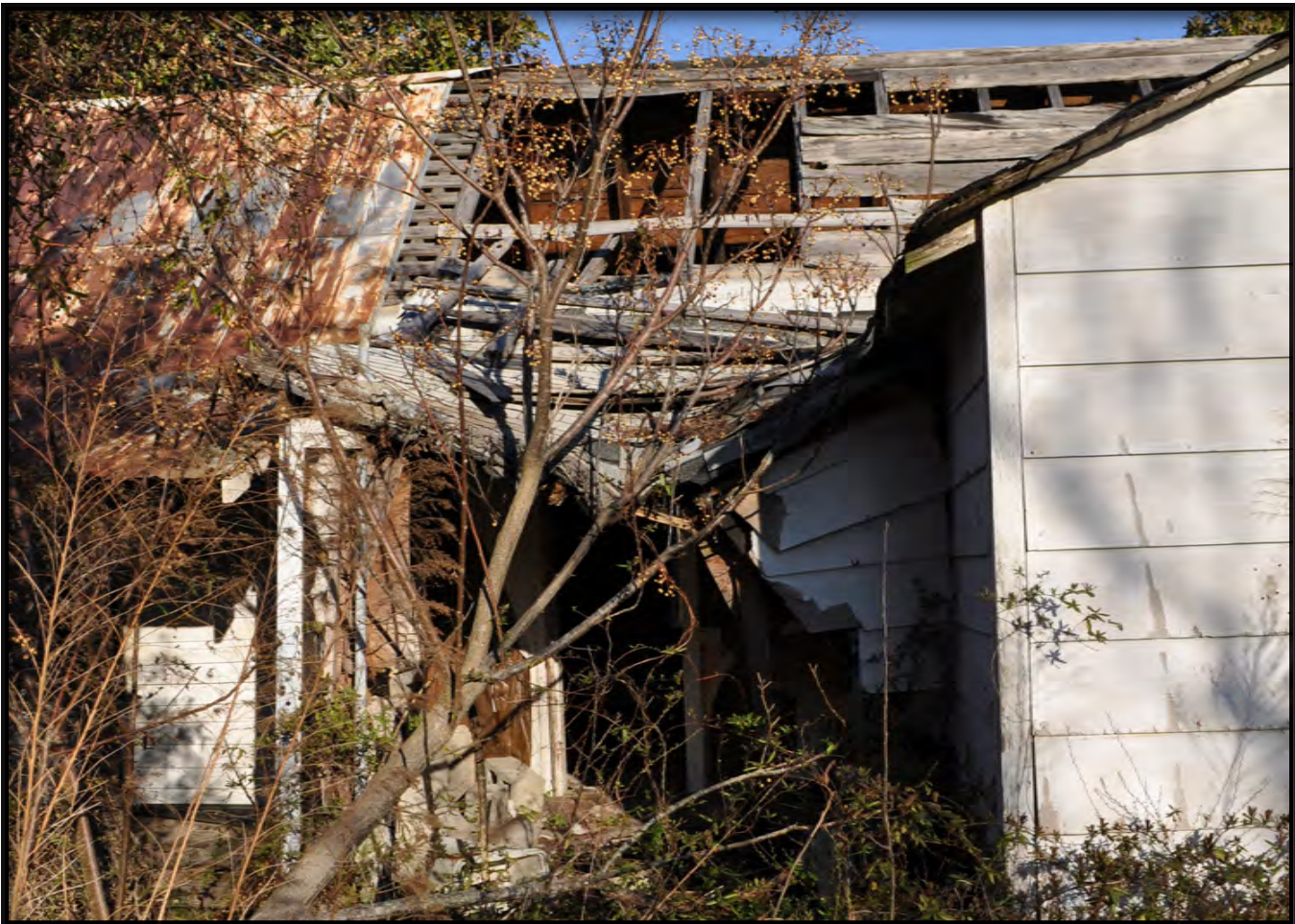
Figure 38. Close-up of West Elevation Showing Porch Collapse
