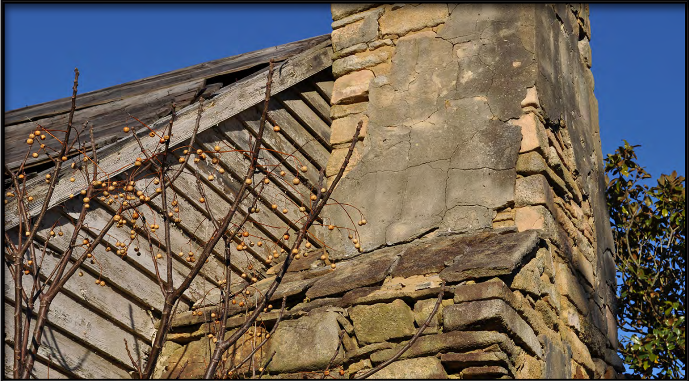
Figure 37. Detail of West Side of Chimney Showing Stone Shoulder Pavers and Remnants of Stucco
