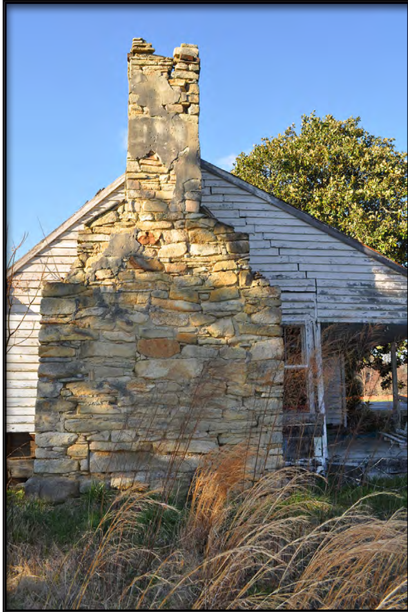
Figure 36. Stone Chimney on South Elevation, Note the Separation of Weatherboards Where Shed Porch has been Added
