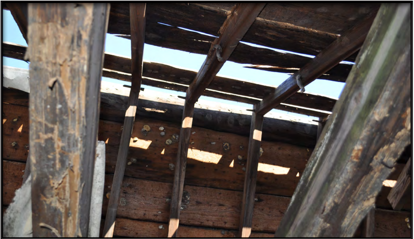
Figure 41. View of Rafter, Pegged Ridge, and Butt Jointed Sheathing in circa 1830s Section
